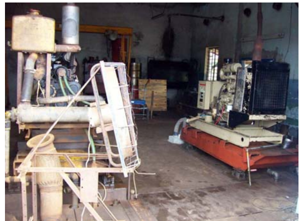
Generators at ELWA
